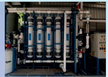
Community Scale Water Purification Plant
