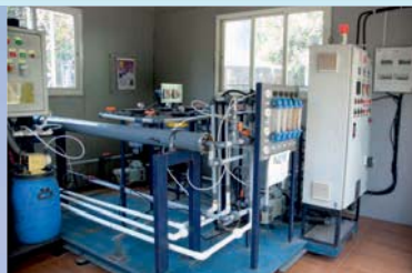
Spiral Ultrafiltration (Uf) Membrane based Community Scale Water Purification Plant
